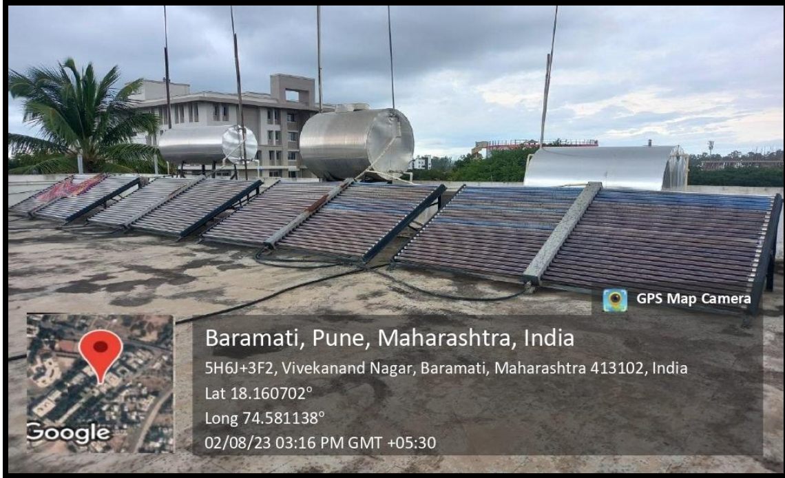
Solar Heater at Rooftop of 'A' Wing of Girls Hostel
