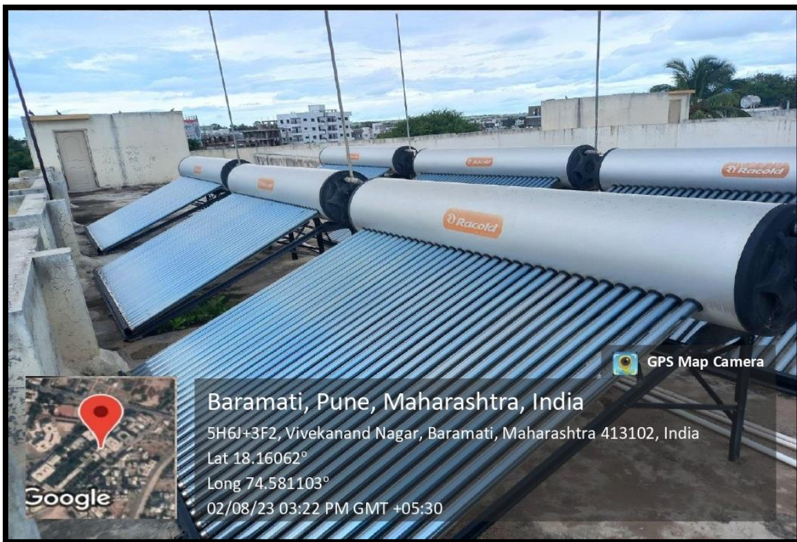
Solar Heater at Rooftop of 'New' Wing of Girls Hostel
