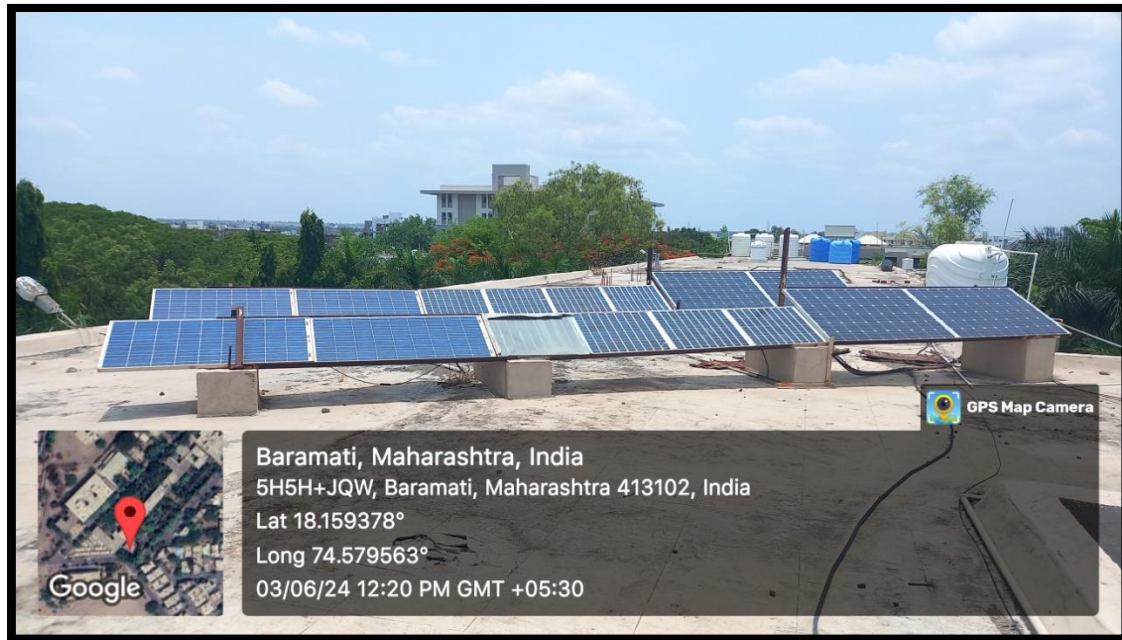
Panel at rooftop of Library with 16 modules
