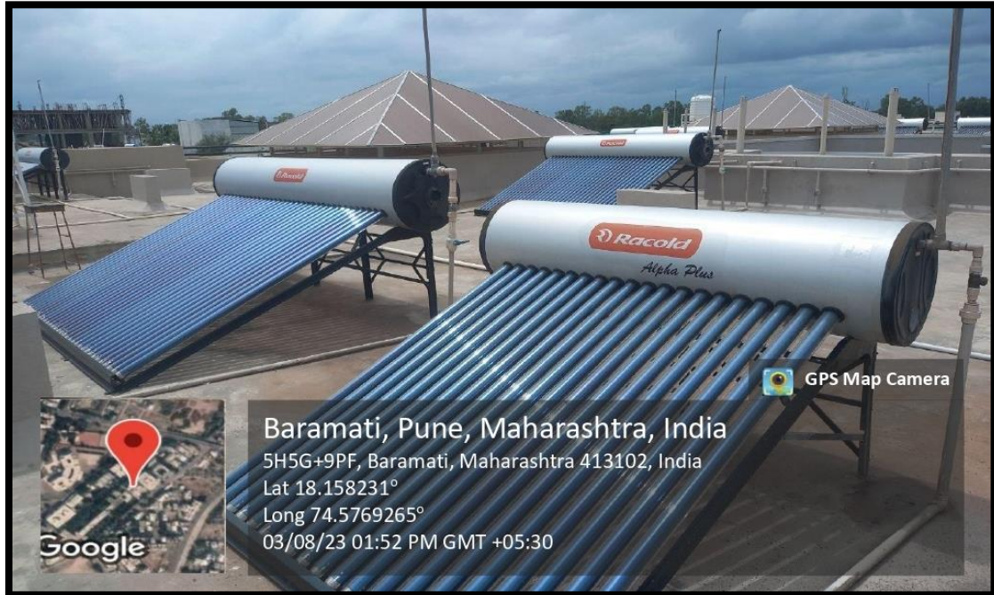
Solar Heater at Rooftop of Boy's Hostel
