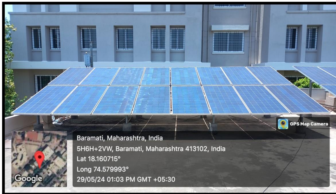
Solar Panel at rooftop of administrative building with 16 modules
