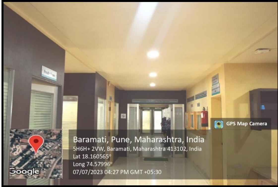
LED lights in Entrance of Computer Science Department
