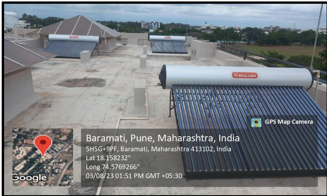
Solar Heater at Rooftop of Boy's Hostel
