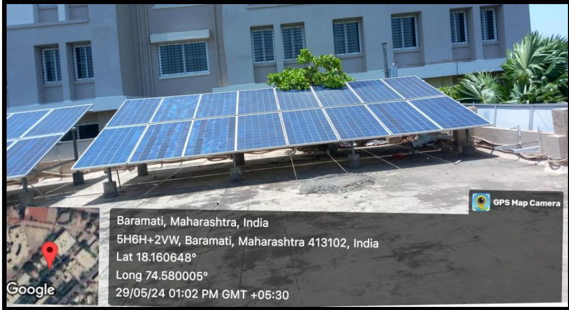
Solar Panel at rooftop of administrative building with 16 modules
