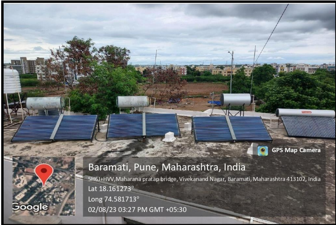
Solar Heater at Rooftop of 'D' Wing of Girls Hostel
