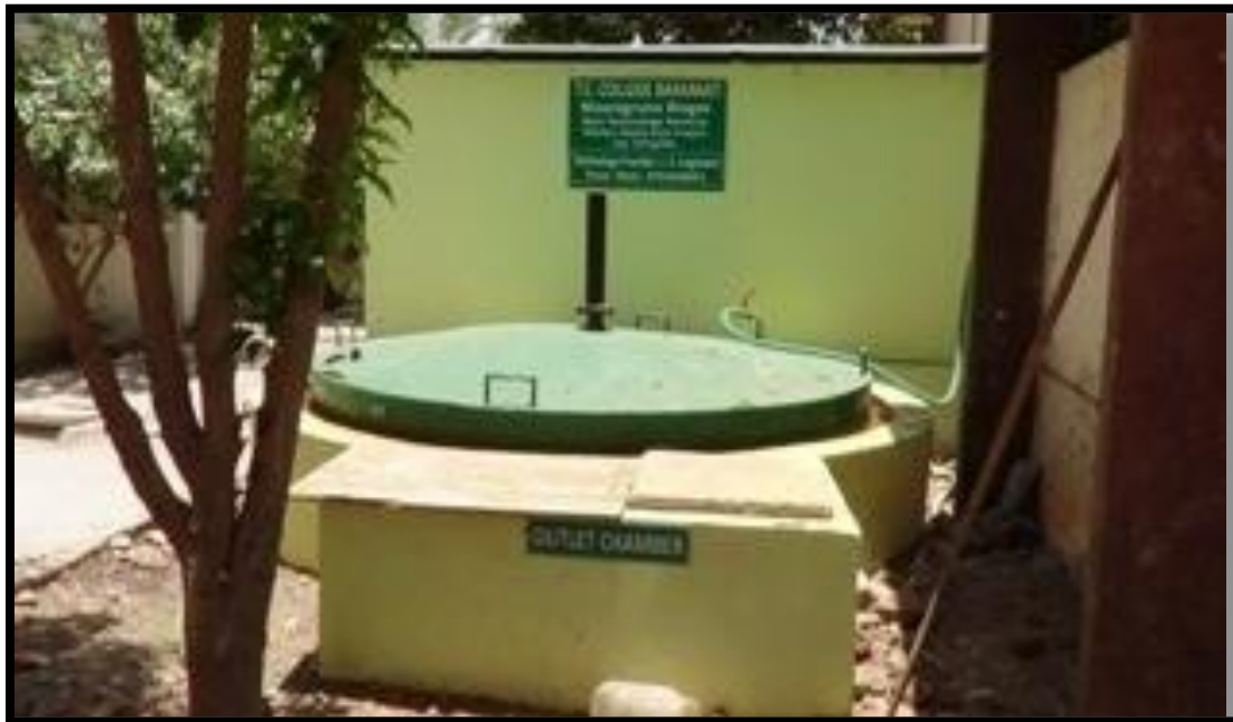
Biogas plant at Girls Hostel
