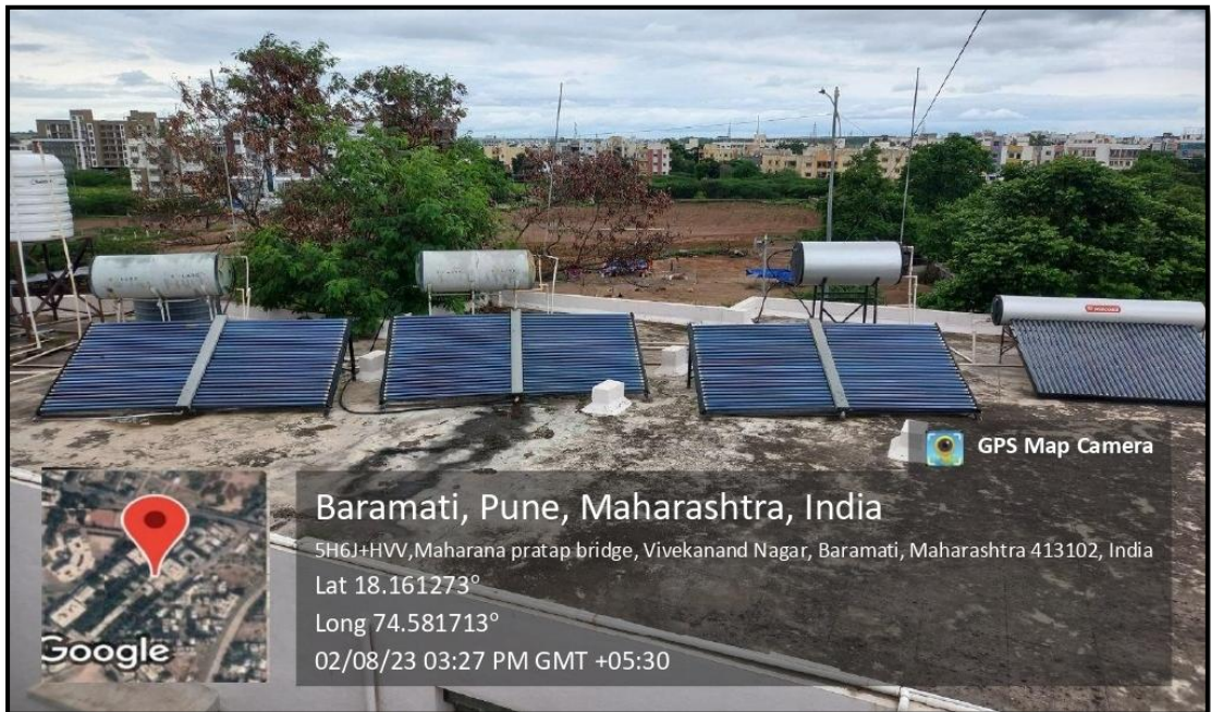
Solar Heater at Rooftop of ‘D’ Wing of Girl’s Hostel
