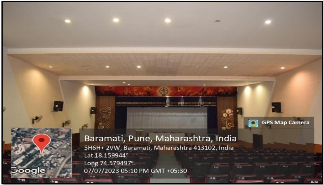
LED lights installed in Auditorum of College- Jivraj Hall
