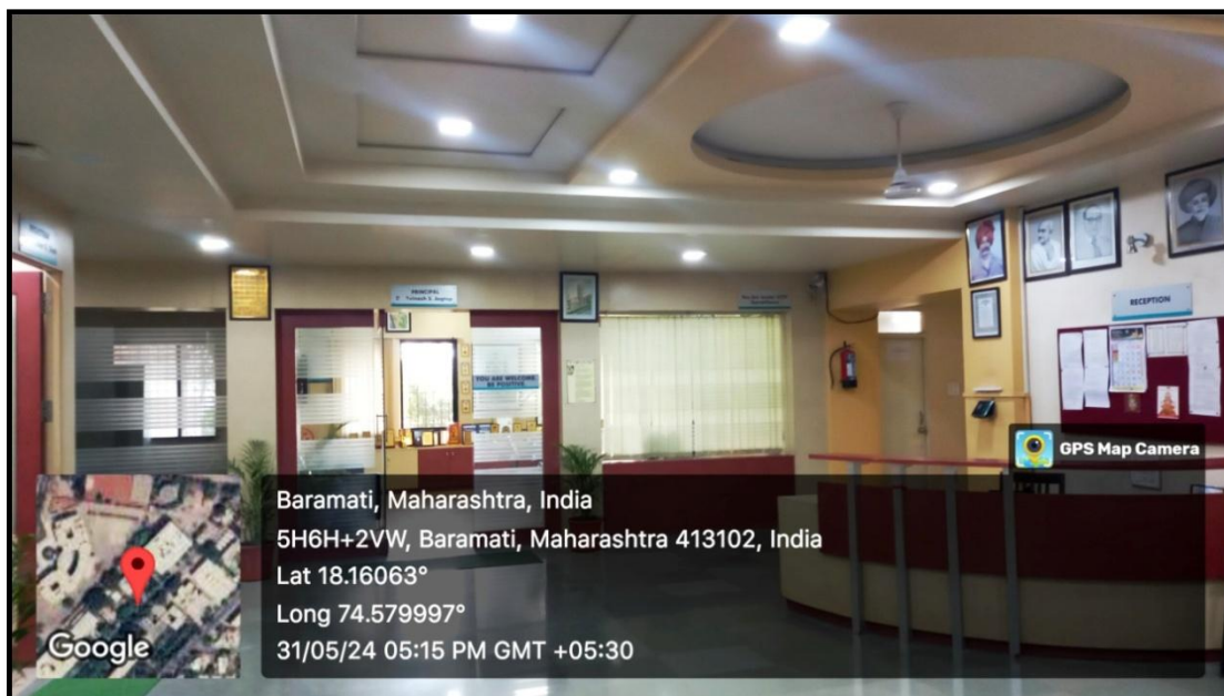
LED panels in front of Principal's office
