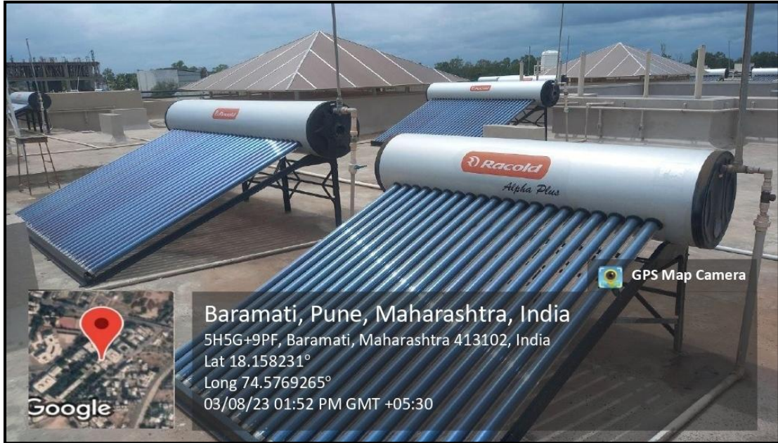
Solar Heater at Rooftop of Boy’s Hostel
