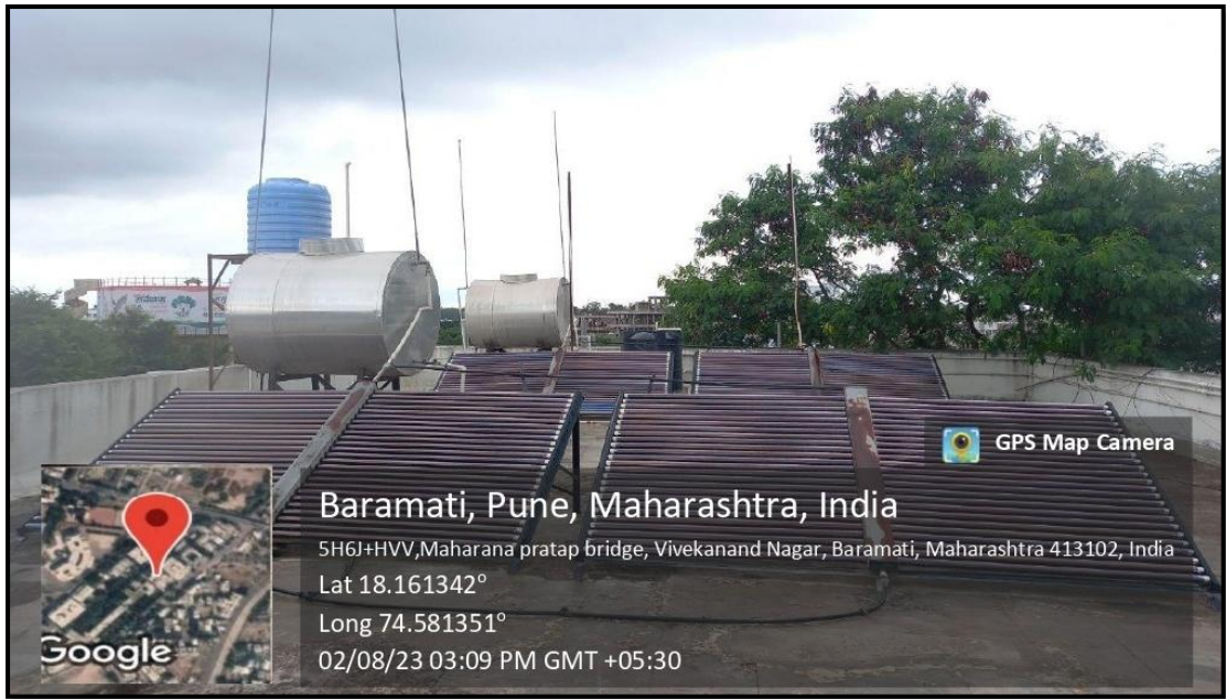
Solar Heater at Rooftop of 'B' Wing of Girl's Hostel
