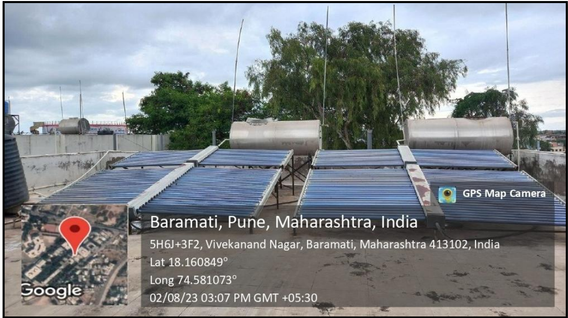
Solar Heater at Rooftop of ‘C’ Wing of Girl’s Hostel
