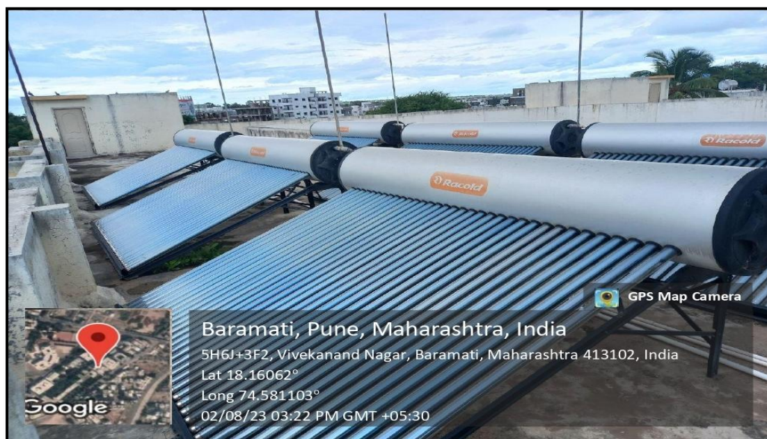
Solar Heater at Rooftop of ‘New’ Wing of Girl’s Hostel
