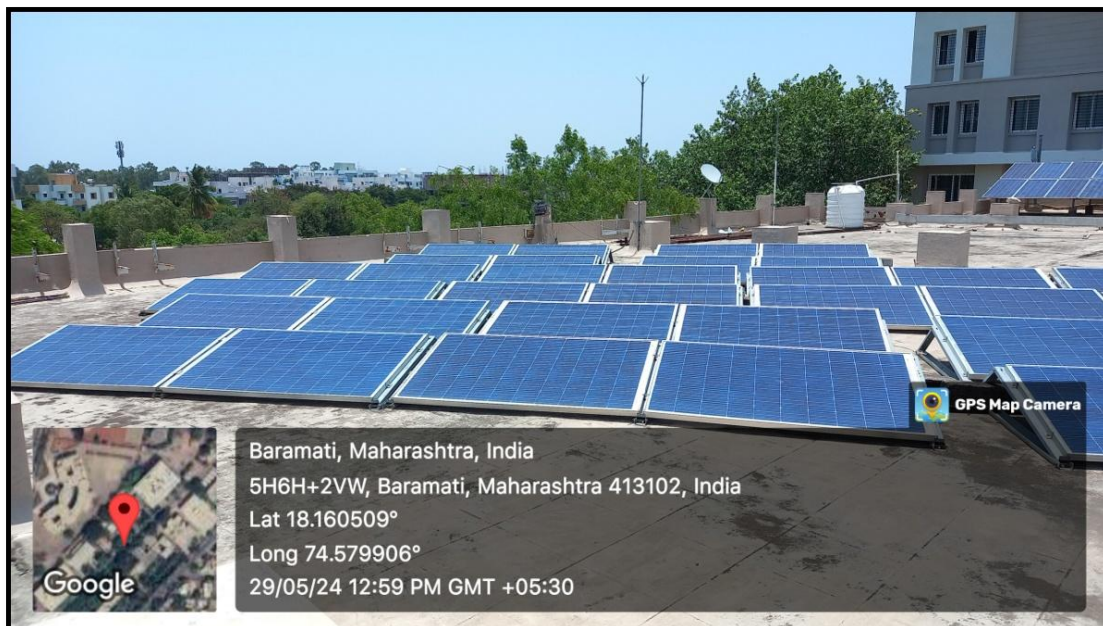
Solar Panel at rooftop of Administrative Building with 40 modules
