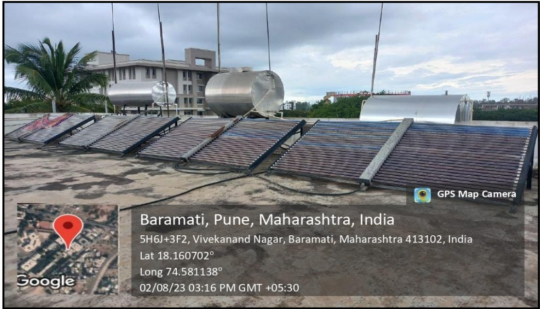
Solar Heater at Rooftop of 'A' Wing of Girl's Hostel
