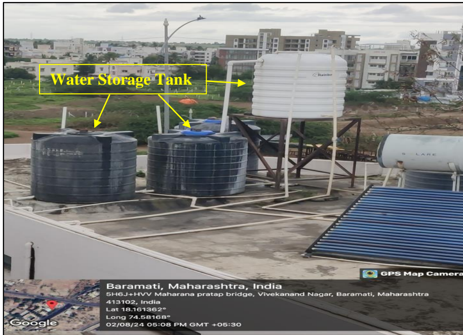
Girl's Hostel: Water Storage Tanks: Storage Capacity 50,000 Lt.
