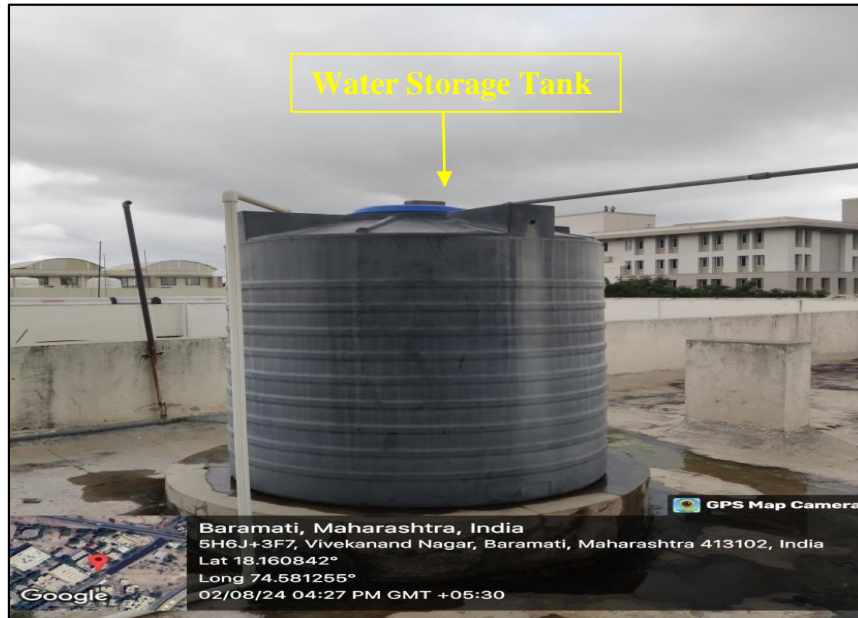
Girl's Hostel: Water Storage Tanks: Storage Capacity 50,000 Lt.
