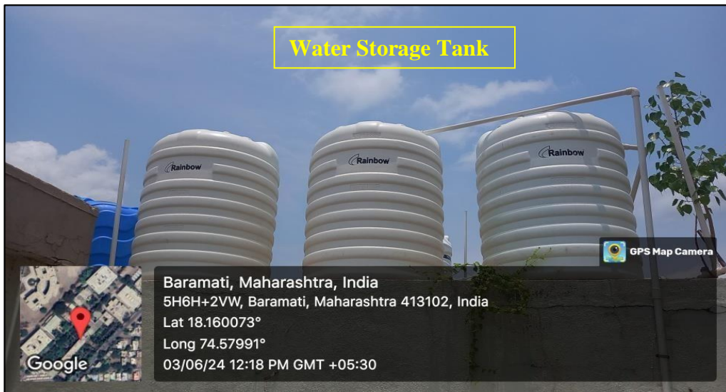
Water Storage Tanks: Storage Capacity 50,000 Lt.
