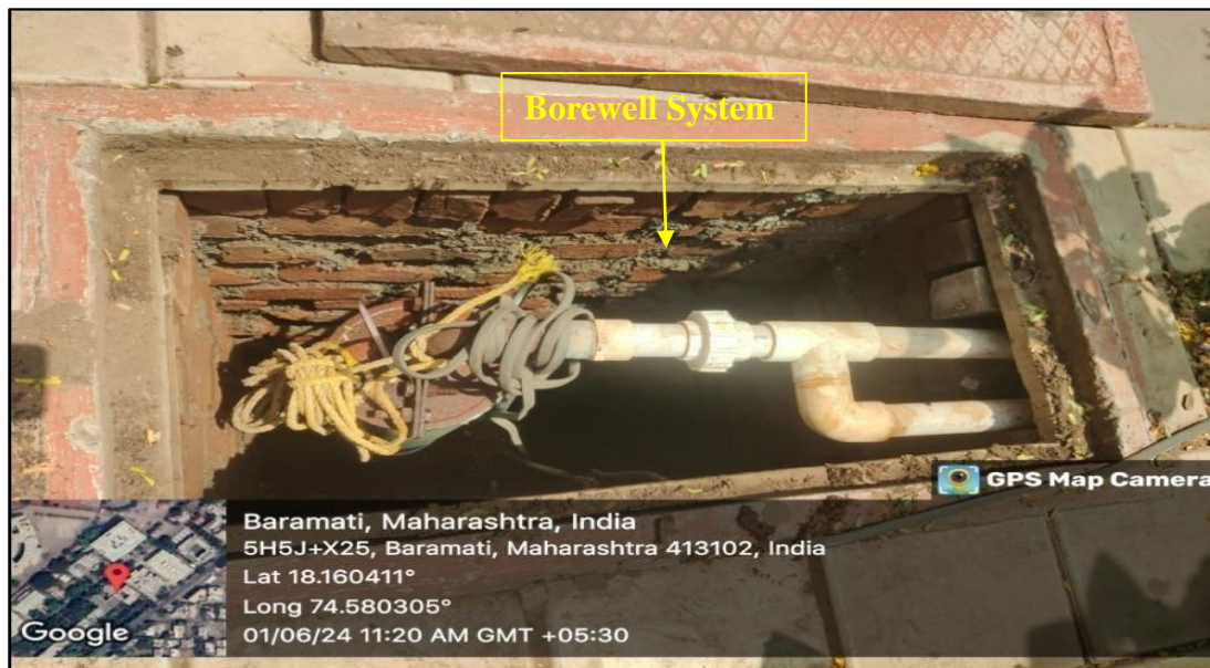
Near Main Building: Borewell System
