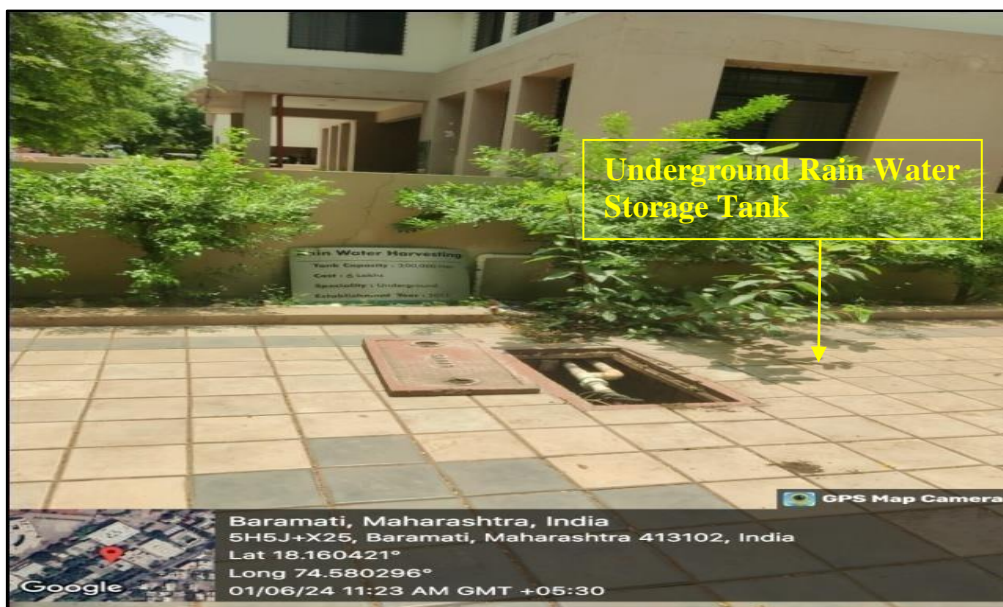
Near Main Building: Rain Water Harvesting System
