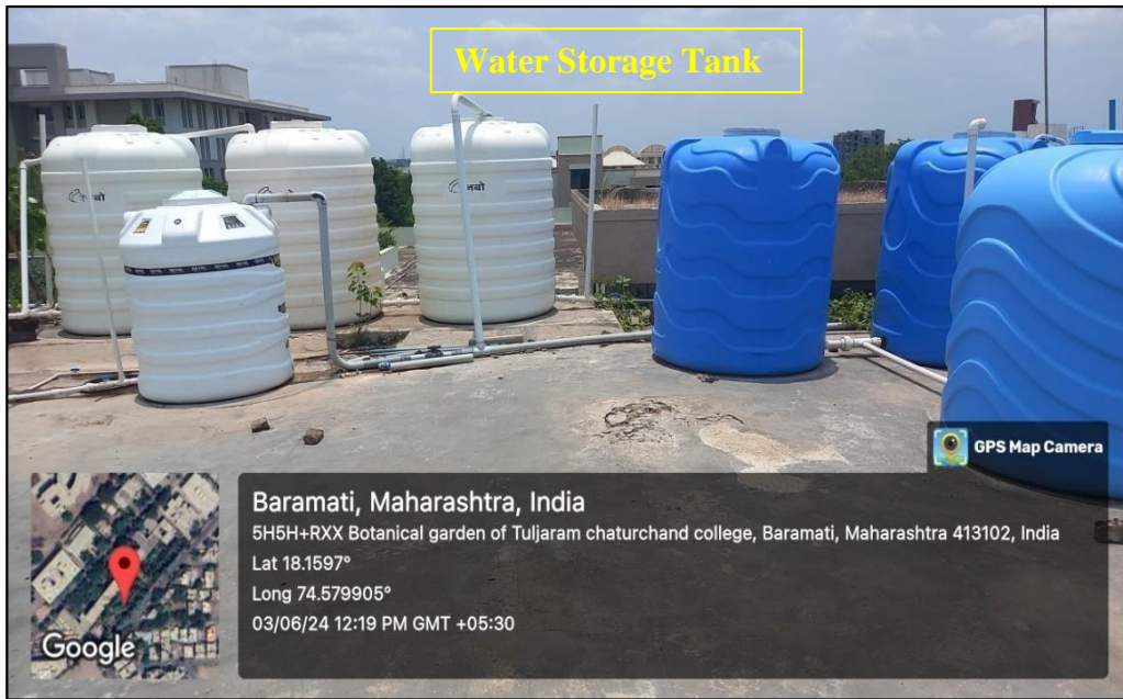
Water Storage Tanks- Storage Capacity 50,000 Lt.
