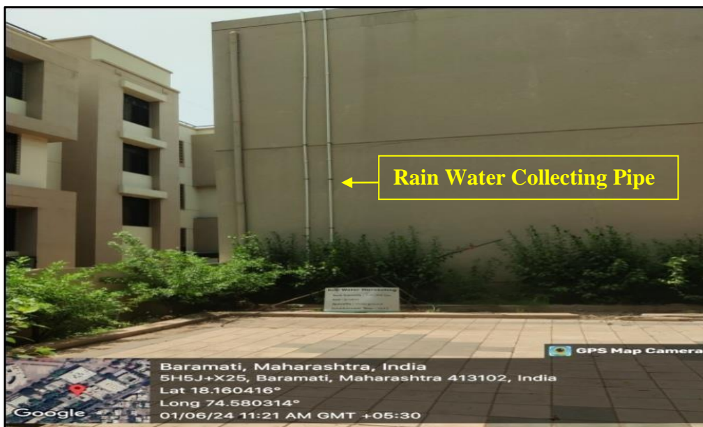
Near Main Building: Rain Water Harvesting System
