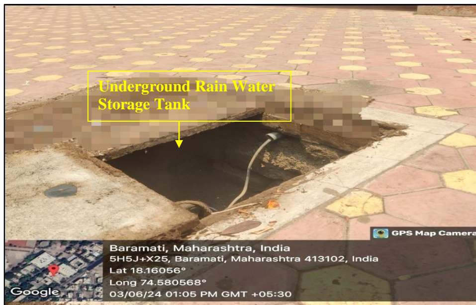
Near Vocational Building: Rain Water Harvesting System
