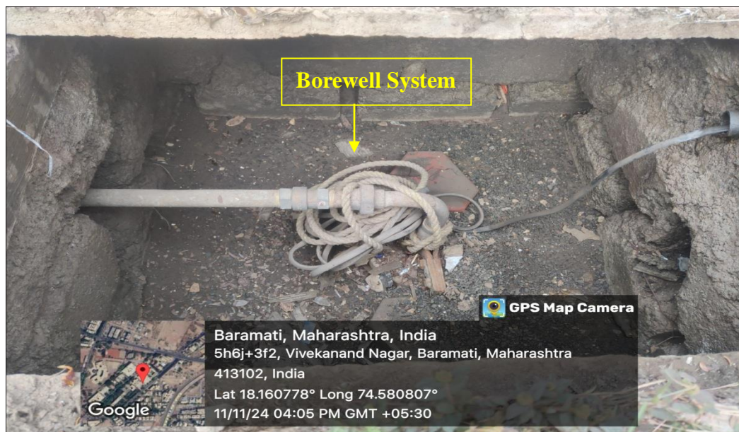
Near Vocational Building: Enclosed Borewell System
