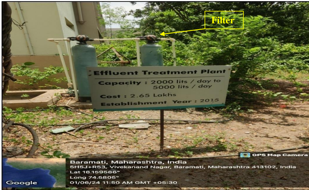
Effluent Treatment Plant System: Capacity 2000 lits /day to 5000 lits /day
