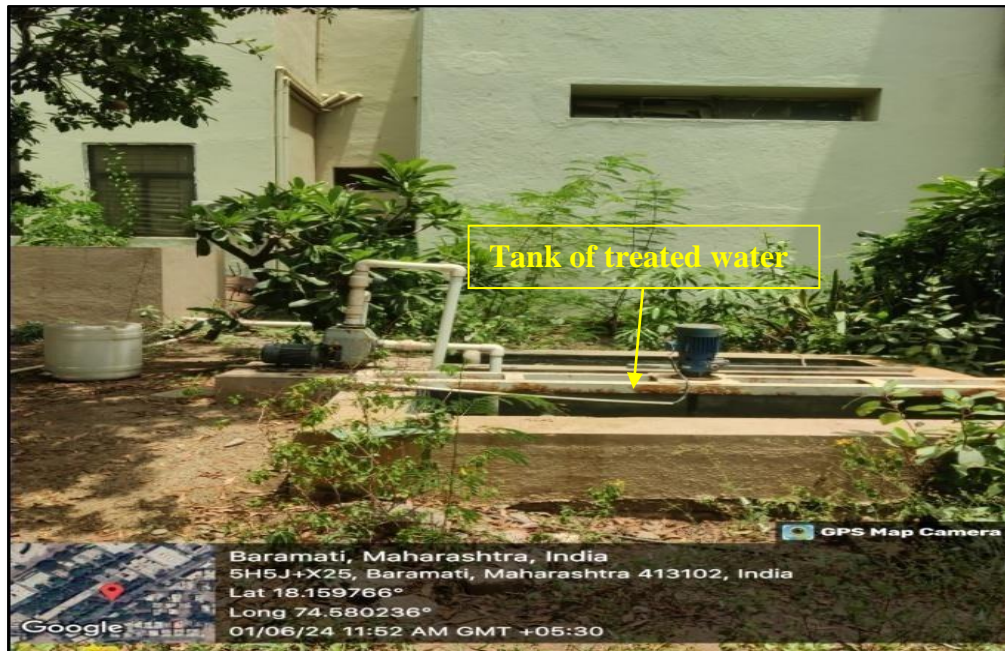
ETP Treated Water Tank
