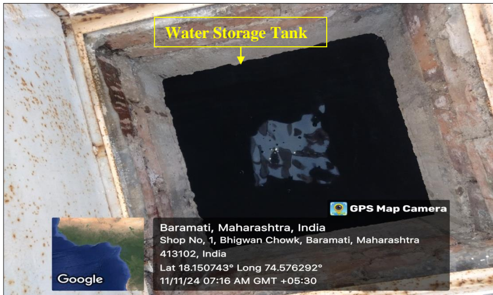
Water Storage Tank: Storage Capacity 50,000 Lt.
