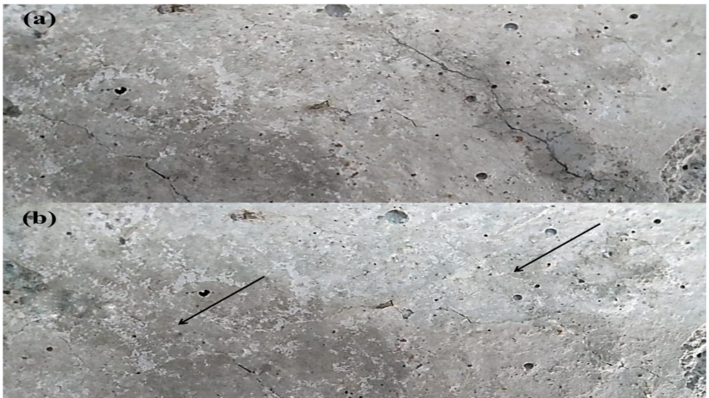
Fig. 5: Remediation of concrete cracks in the cement mortars. (a) mortar cracks seen on 0 day (before treatment); (b) calcite filled cracks indicated by solid arrows 14 days post-injections with cementation solution containing Bacillus cereus SSS1 bacterial suspension
