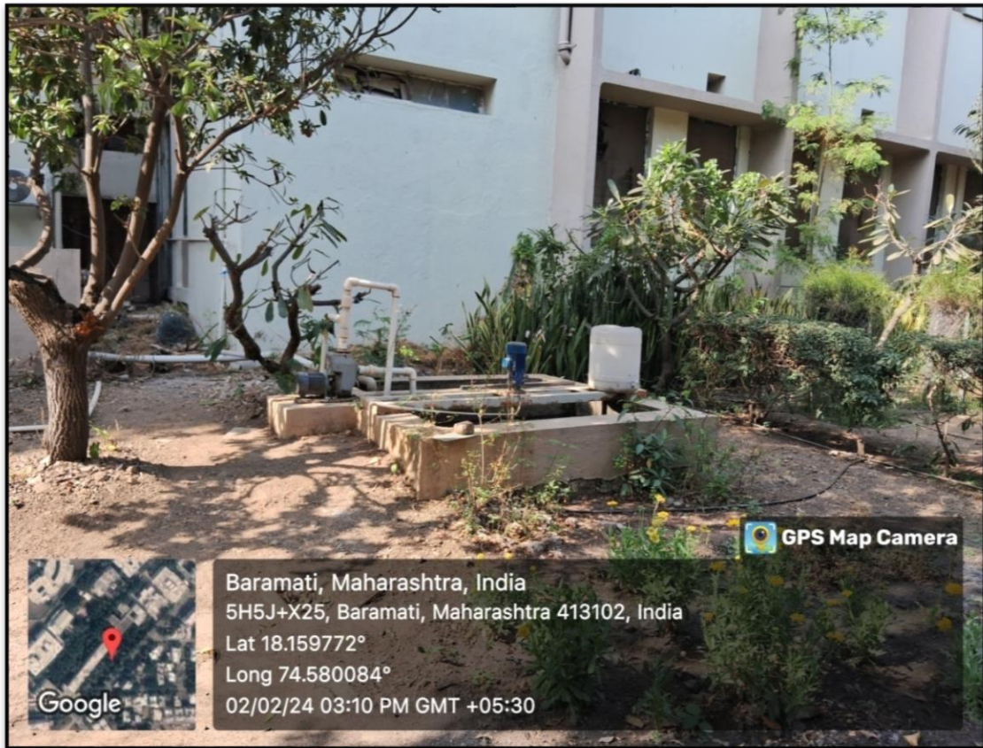
Effluent Treatment Plant (ETP): Effluent collection and processing pits
