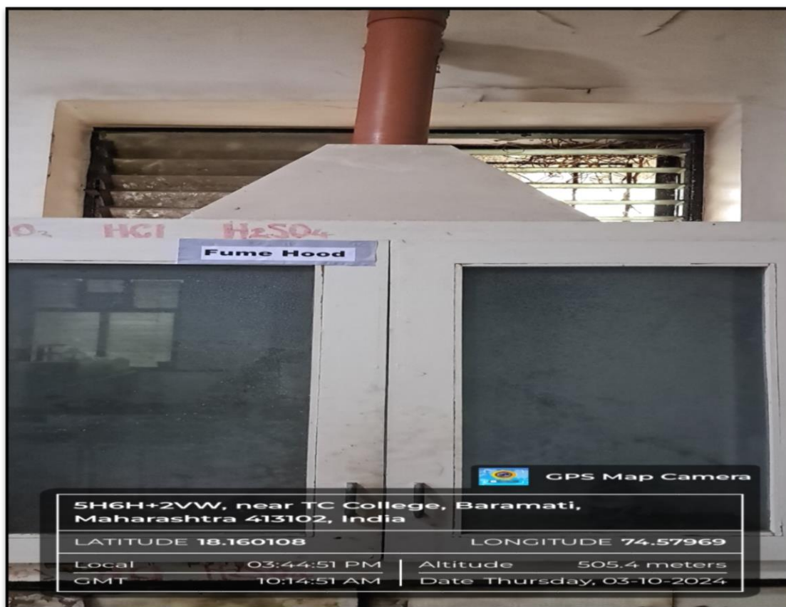
Fume Hoods and Safety Equipment at chemistry laboratory
