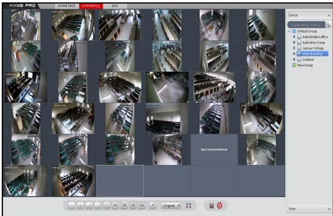
Centralized CCTV Surveillance Monitoring
