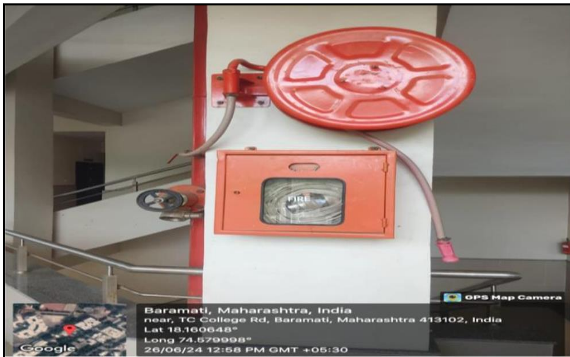
Fire Safety System
