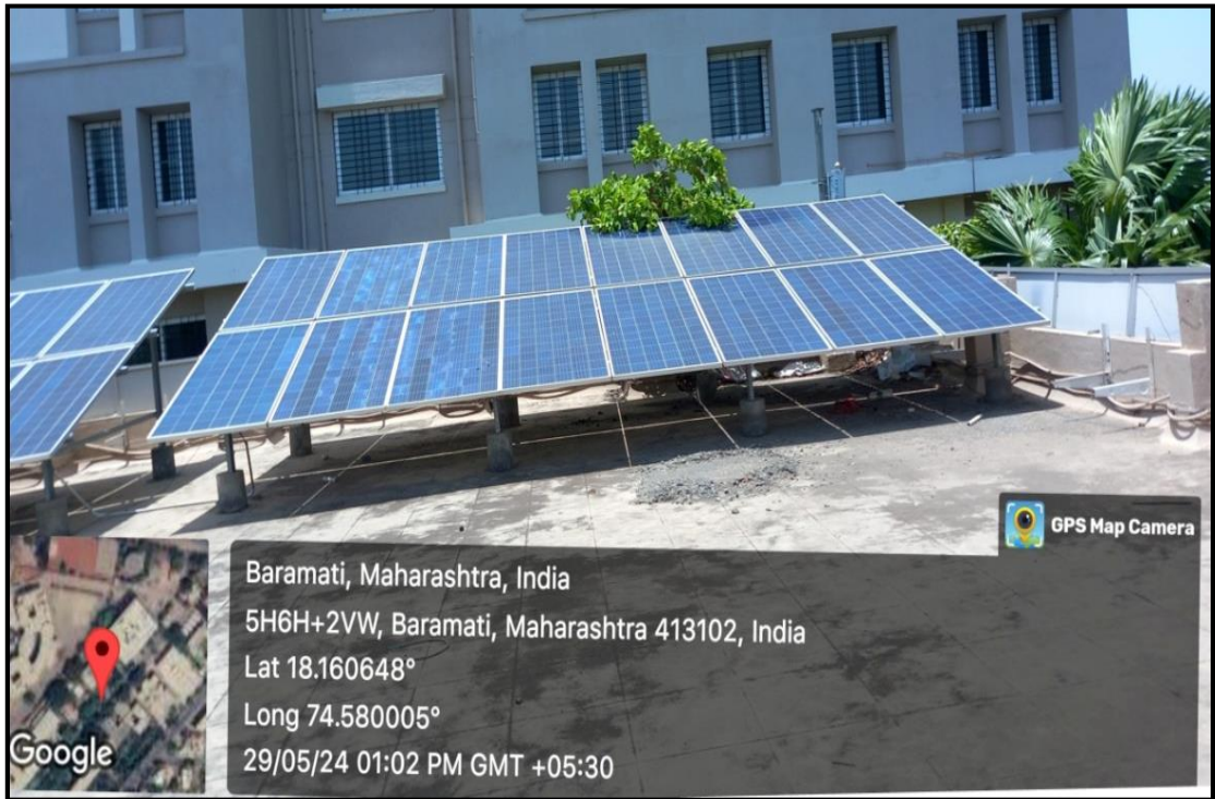
Solar Panel at rooftop of administrative building with 16 modules
