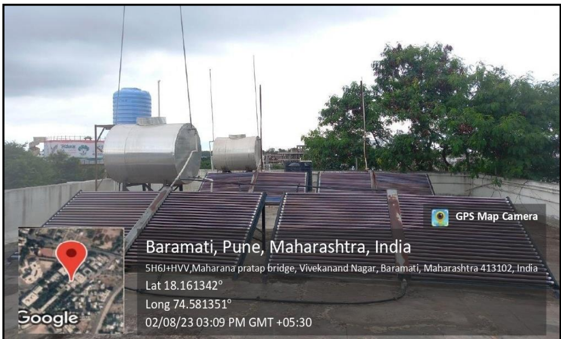
Solar Heater at Rooftop of 'B' Wing of Girls Hostel
