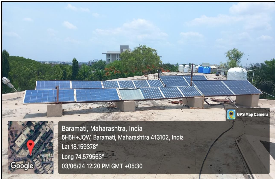
Solar Panel at rooftop of Library with 16 modules
