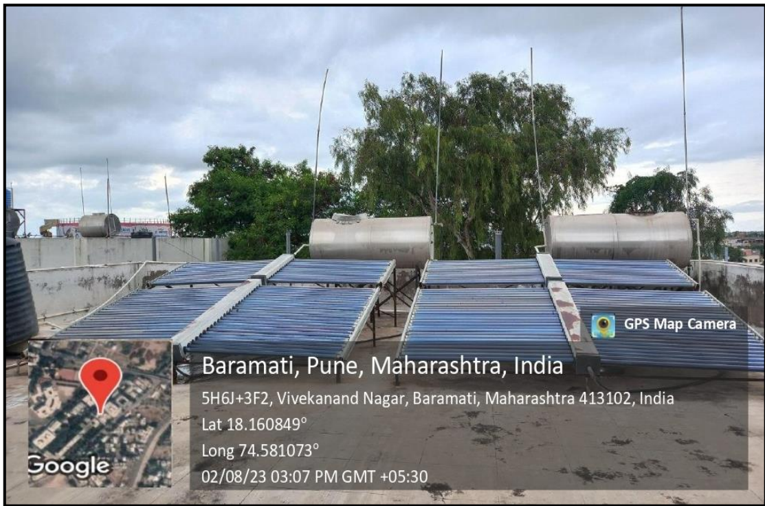
Solar Heater at Rooftop of ‘C’ Wing of Girls Hostel
