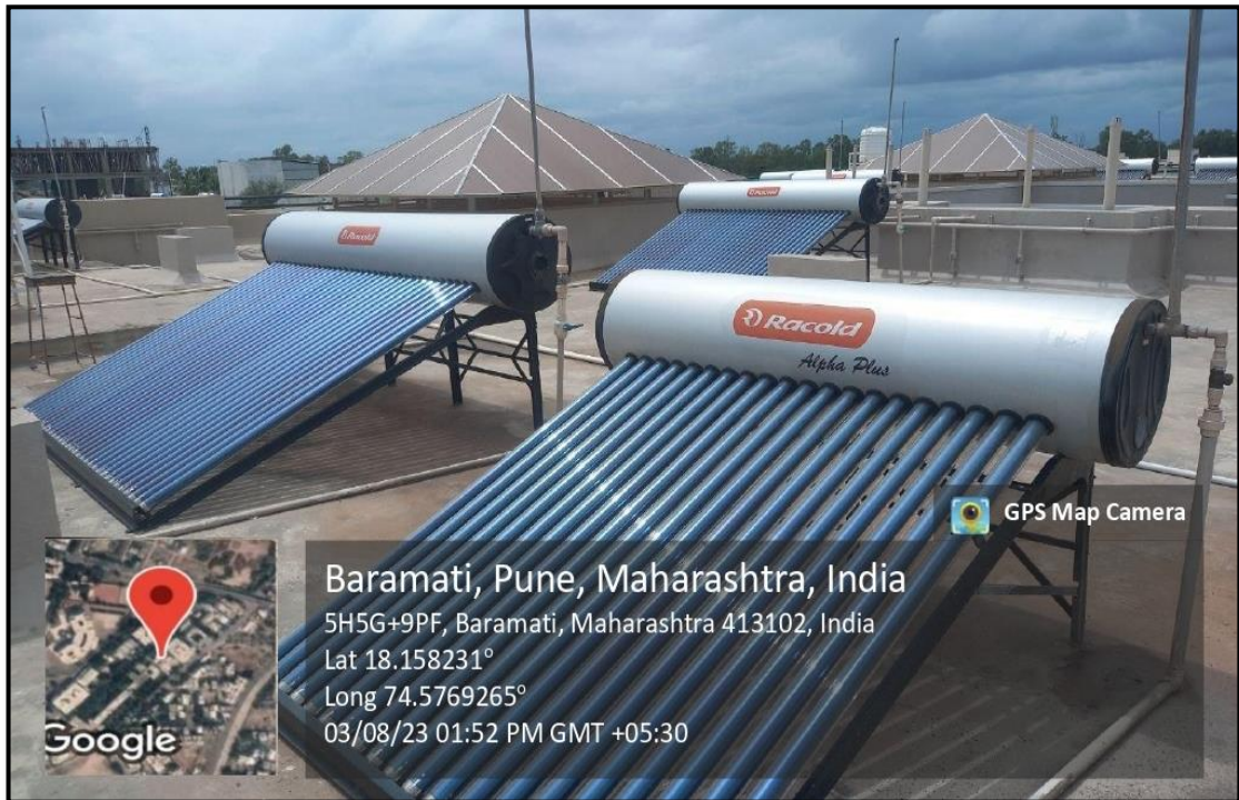
Solar Heater at Rooftop of Boy's Hostel
