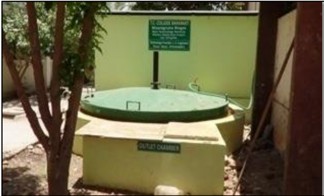
Biogas plant at Girls Hostel
