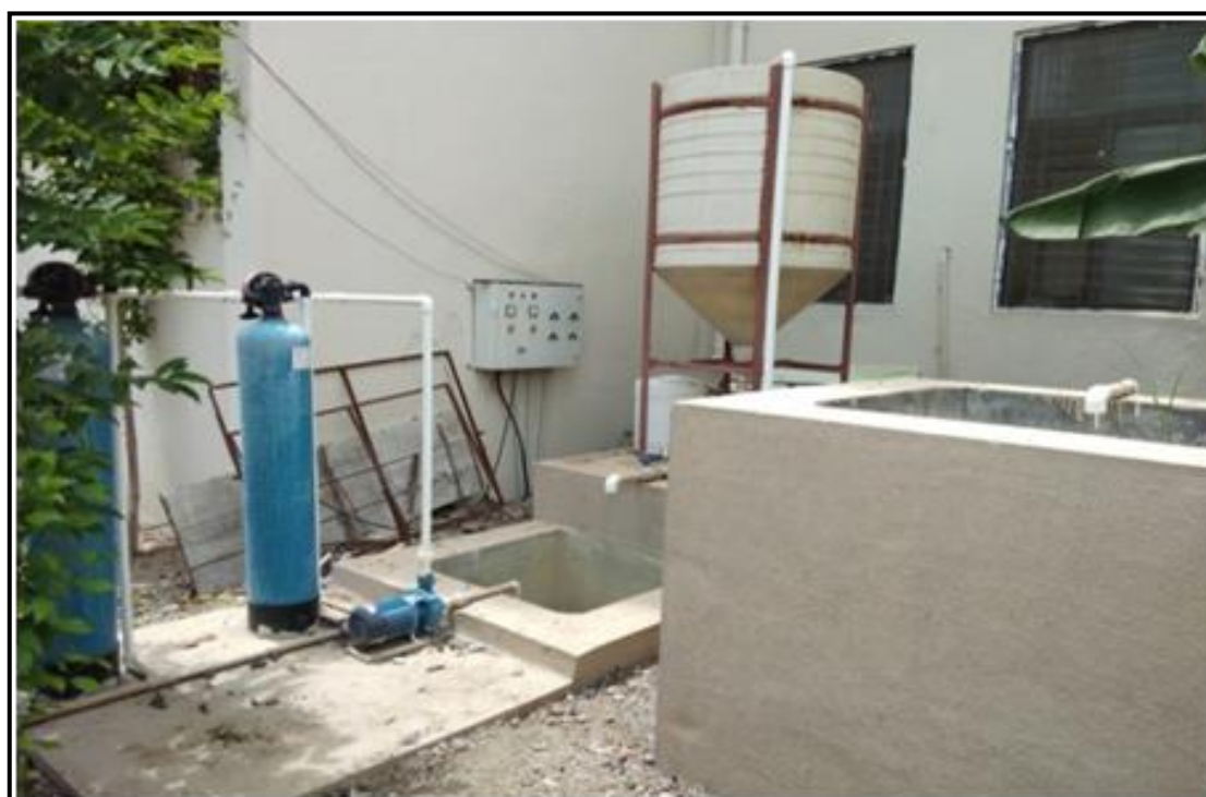
Effluent Treatment Plant in the college garden
