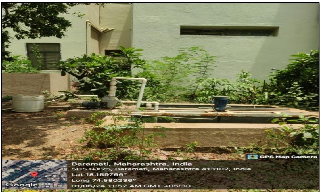
Geo-tagged photos of Effluent Treatment Plant of the college
